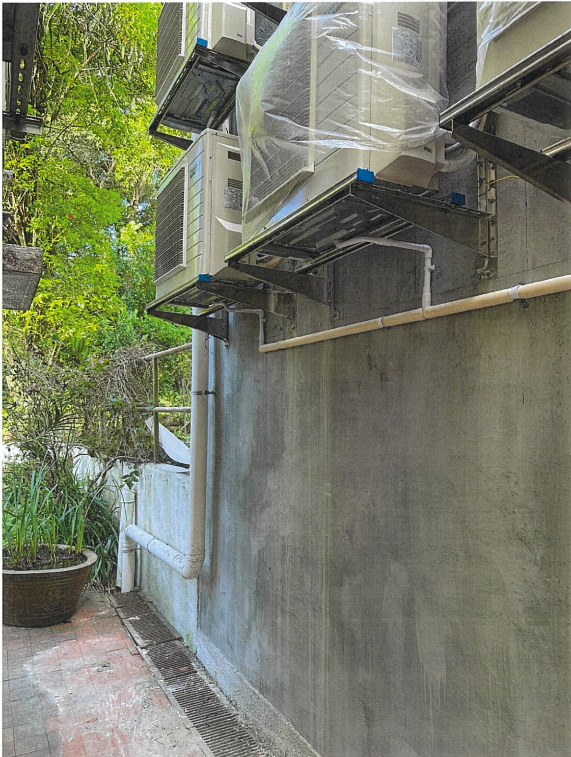
Picture 6 shows the extended drain pipe
