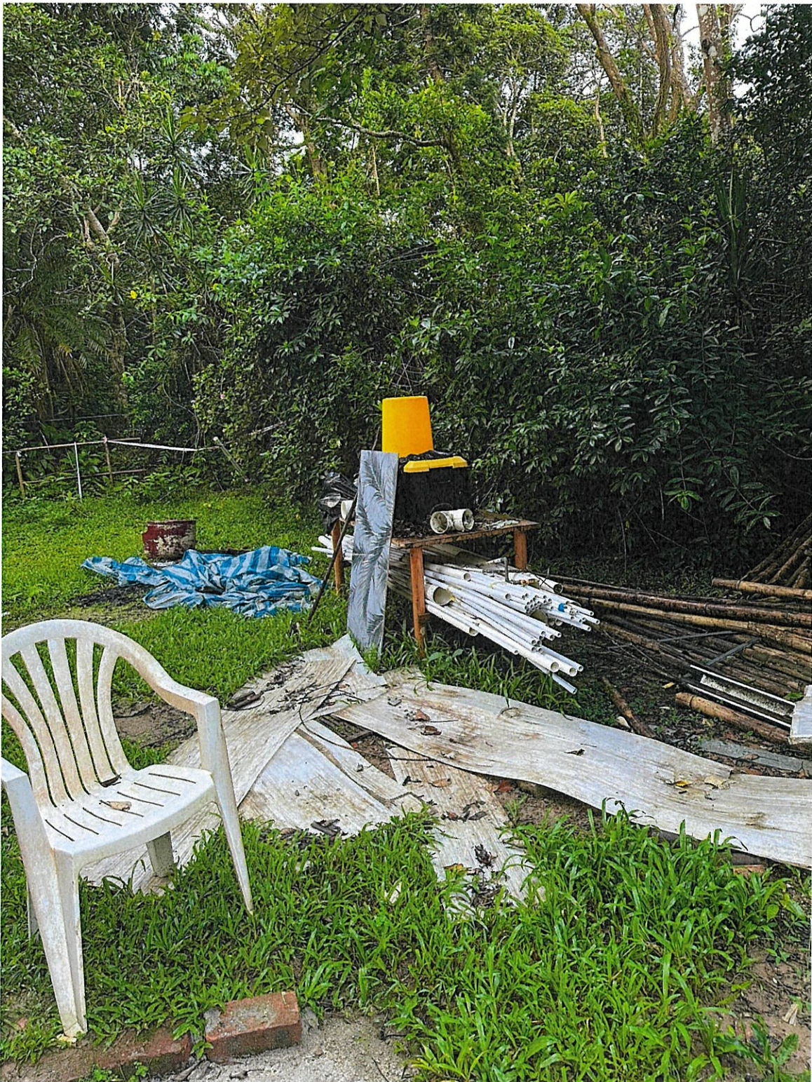
Picture 7 shows the multiple uninstalled pipes
