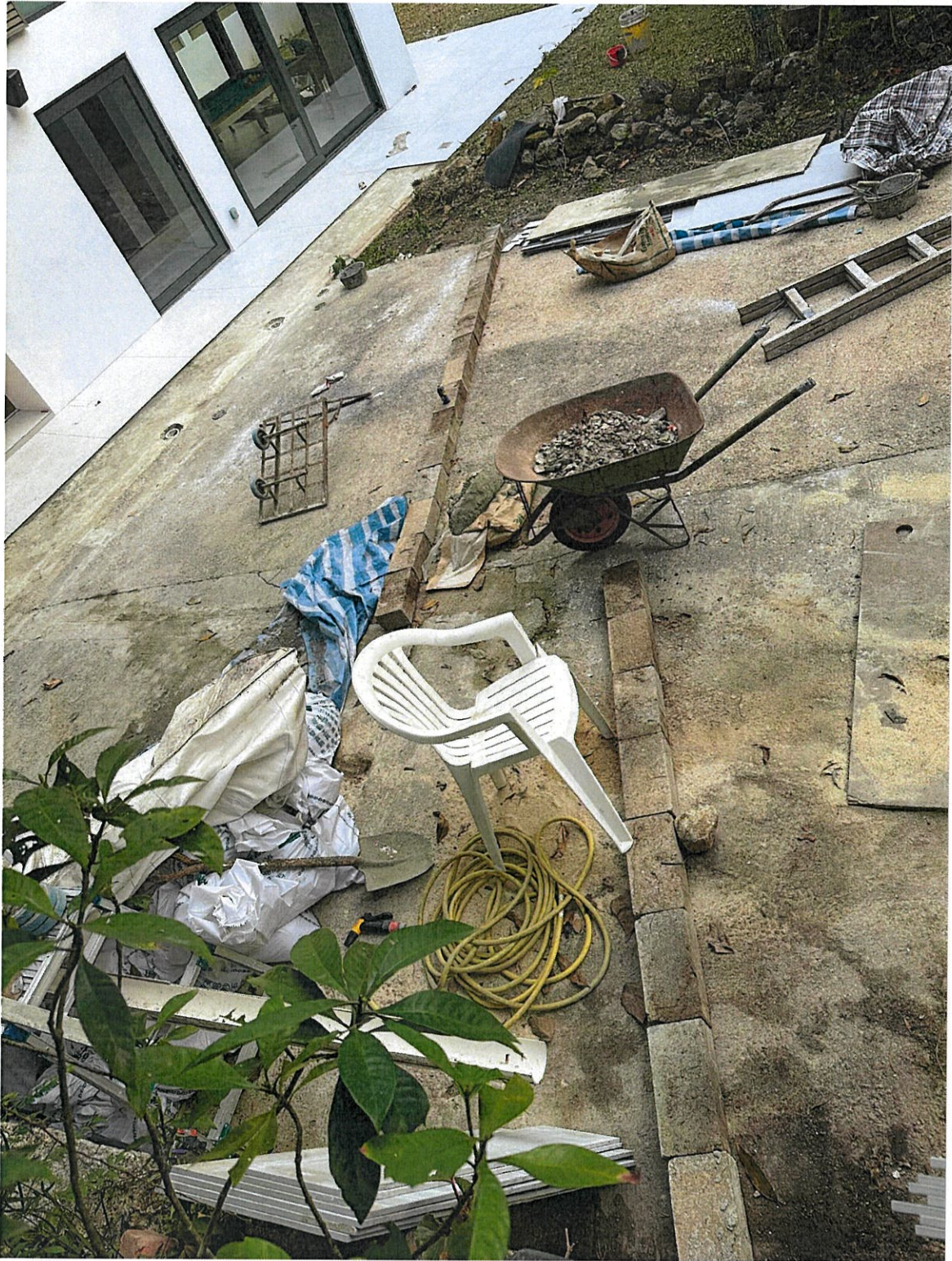
The photo shows the bricks marked out to direct rain water to drainage.
